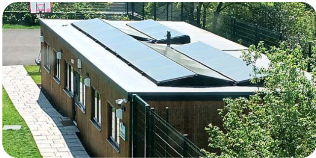
Castlefell School Solar panels installed
